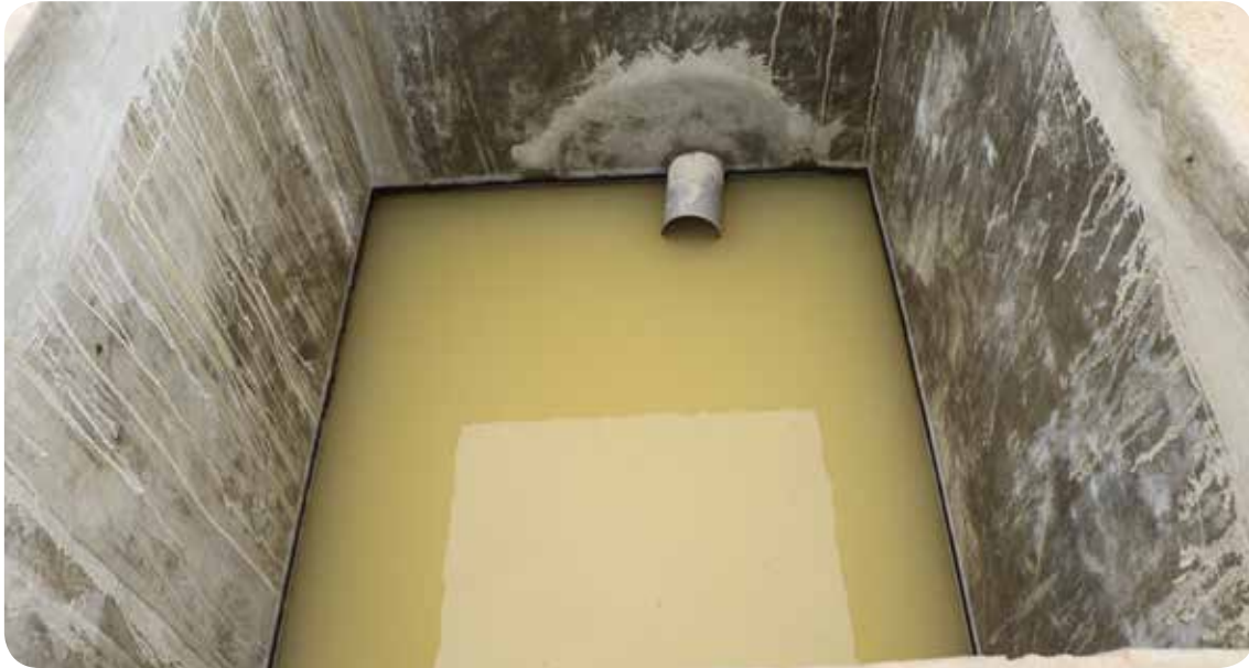
Waste Recycling plant built through a partnership between REMA and Rwanda Correctional Services
