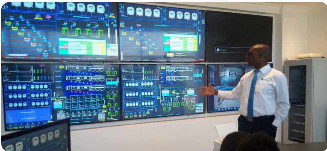
Eng. Aime Muzola, CEO WASAC, explaining the water distribution system in Kigali
